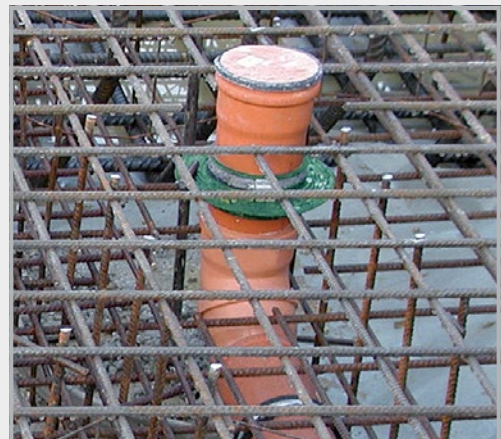
The RONDO, shortly before placement of concrete. The drainpipes are securely and permanently sealed against rising moisture.
